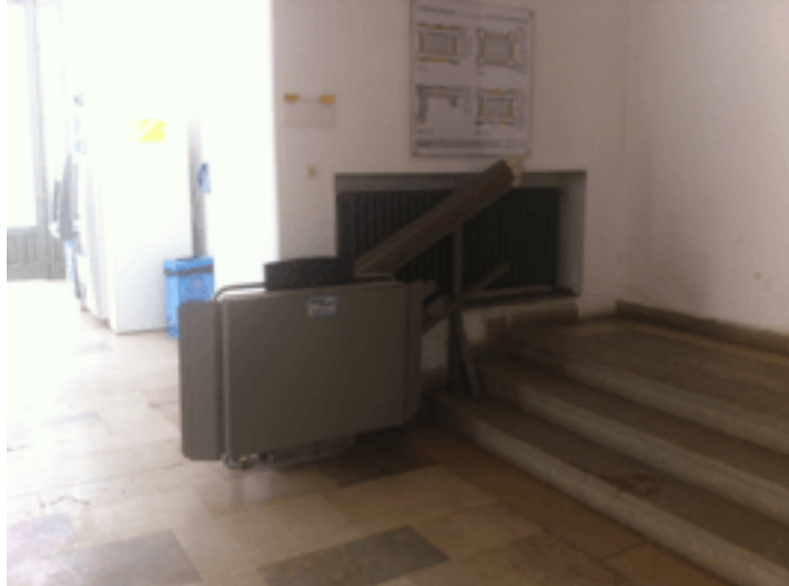
Figure 1.11: Ground floor disabled elevator
