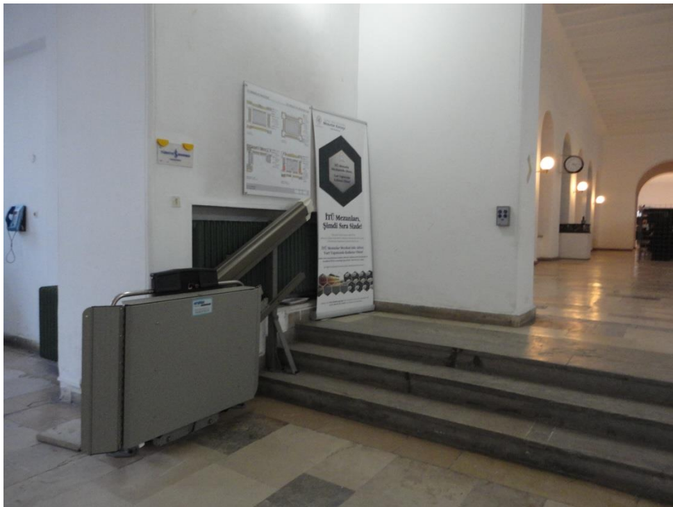
Photograph of one stair-lift
